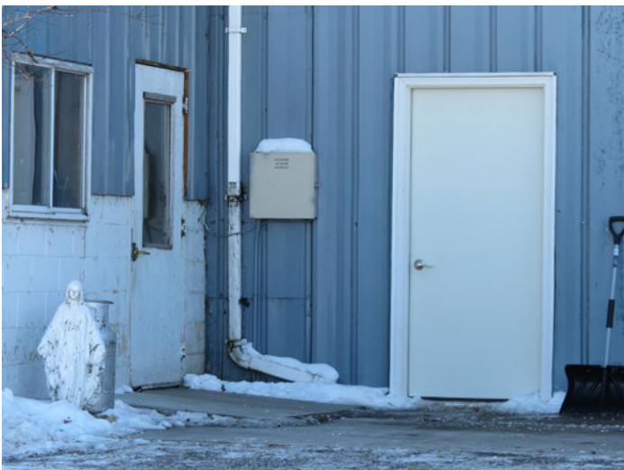
Figure 22. Service doors 36-inches wide with lever handles as shown are easy to open for all workers. Ramps should meet ADA standards with 12:1 slope and 1/2" thresholds.
