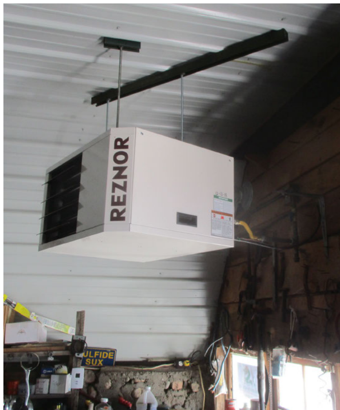
Figure 14. This well-insulated farm shop has gas heat. Fire resistant metal wall material should be installed around heat sources.
