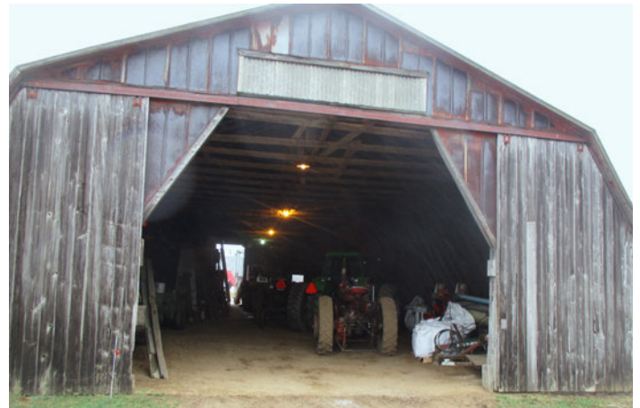
Figure 5. Renovating an existing building may be the only good option from a financial perspective, but upgrades can be very expensive.
