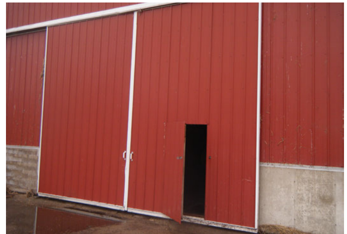
Figure 21. Sliding doors are low cost but may be hard to open and block other parts of the building. A walk-through door designed in the sliding door can allow personal access without opening the heavier large door.
