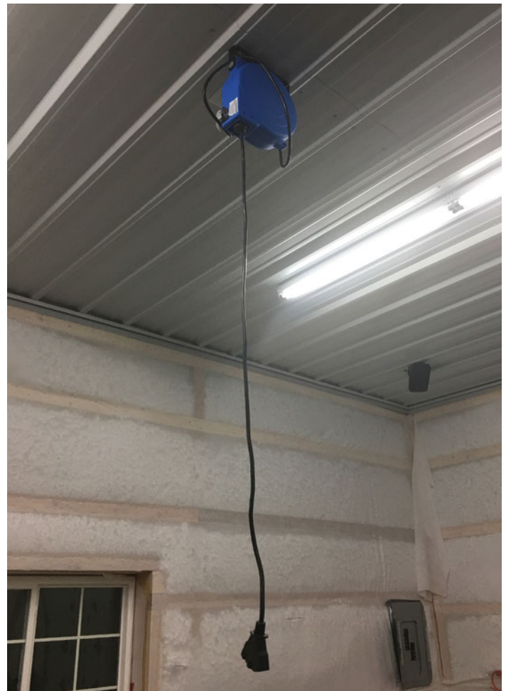
Figure 24. LED is most efficient light source currently available, does not have a "strobe effect", and has a wide operating temperature range. Note the wall insulation and the auto-rewind electric cord to reduce tripping.
