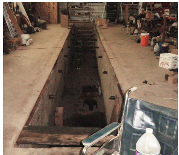
Figure 31. Planning for a service pit, lift or hoist is required during the initial planning and construction of the building to complete excavation and place anchor points.
