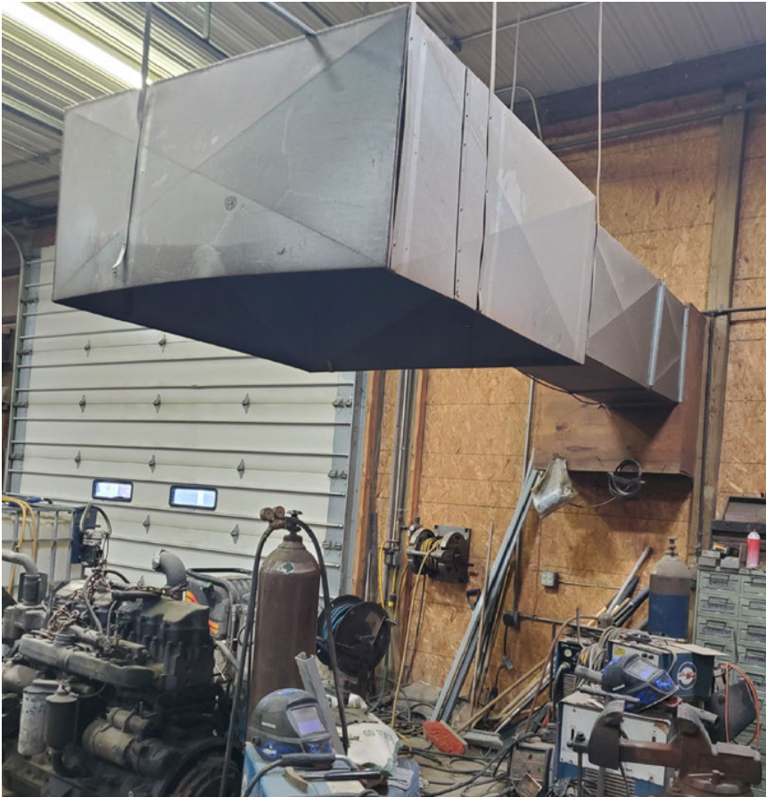
Figure 16. Ventilation hoods can be mounted over the metalworking workbench, or flexible ventilation tubes moved to those sites where welding is going to be done.
