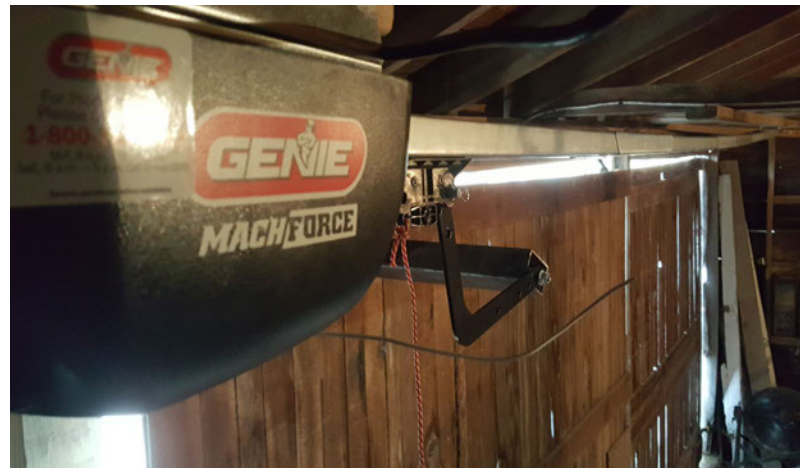
Figure 19. Standard garage door openers can be adapted with custom brackets to open sliding doors.
